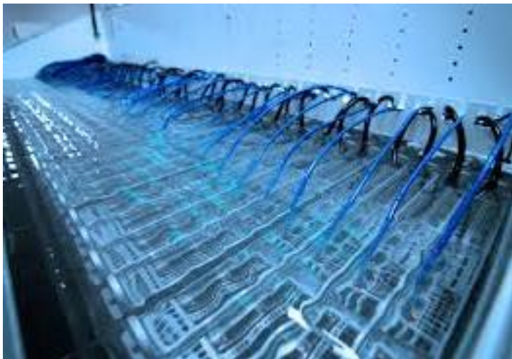
Liquid Immersion Cooling (Image Source:)
